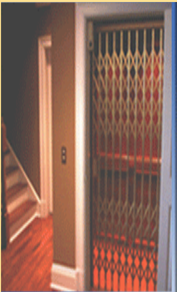
Figure 3: Scissor gate; photo courtesy of Bella Elevator, LLC
